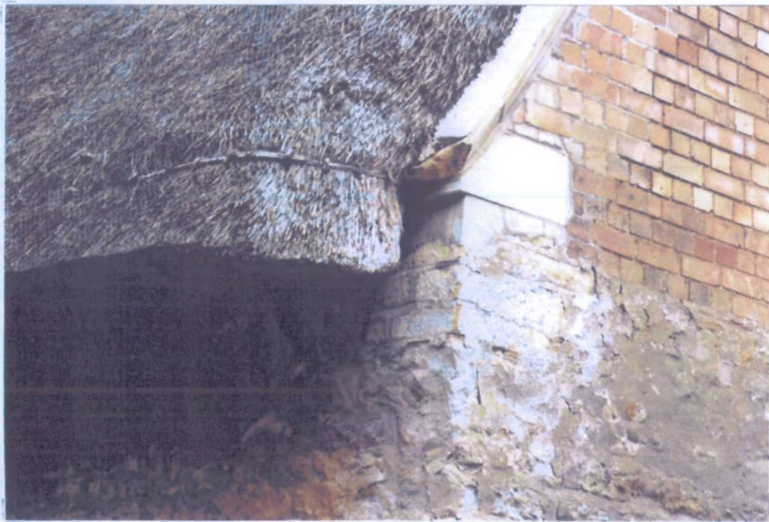
FIGURE 2: DAMAGED REPLACEMENT COPING STONE
